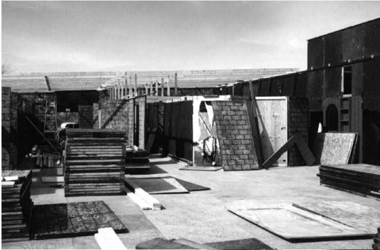
Long shot. To the right is the back of the Grand Entry. Center top is the roof support structure. Center is the central corridor. Assorted panels populate the deck awaiting final placement.
